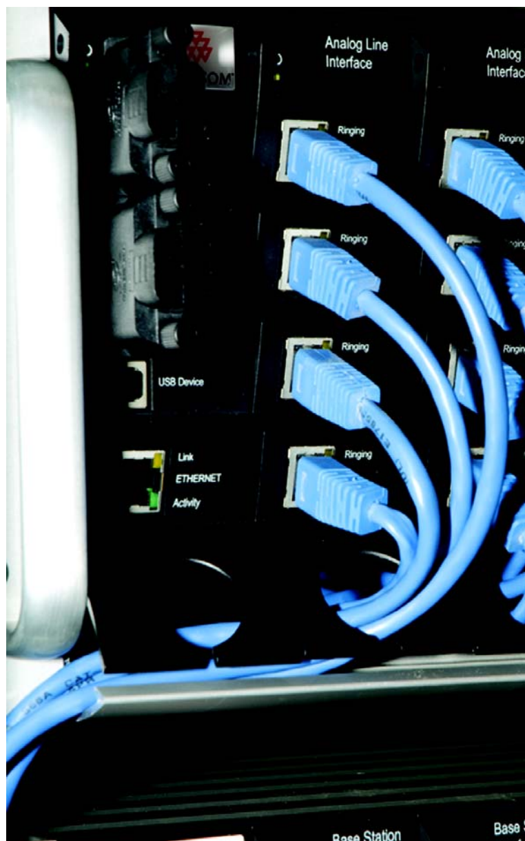
Figure 11 Harnessing cables to the side and out.
