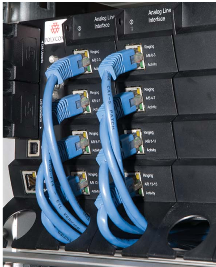
Figure 11 Harnessing cables to the back and out
